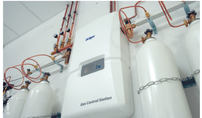
The number of gas cylinders and the fluid gas container sizes may be individually adjusted.
