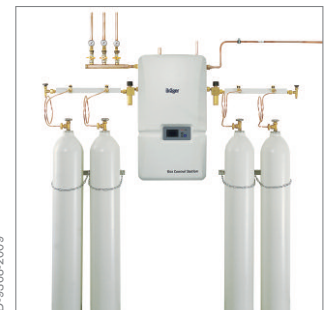
Gas Control Station Example of an oxygen supply facility.
